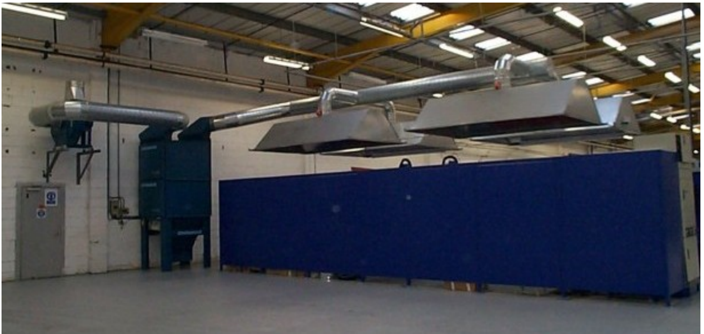
4 – Rear of the cell showing the blanked off stations and integral extraction system
