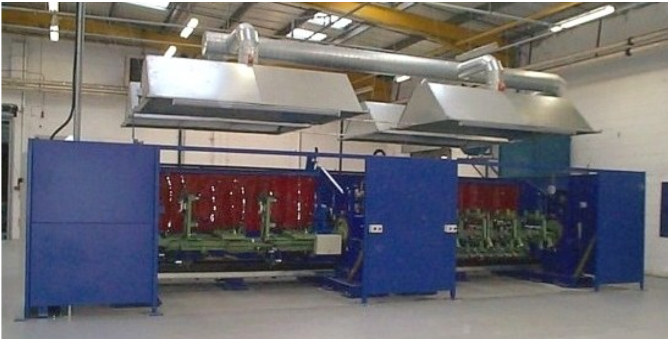
1 – General view of the cell showing the initial weld stations with double sided jiggging
